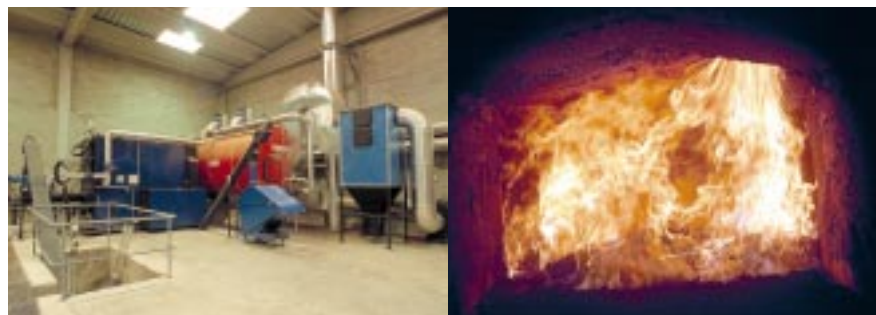
View of the biomass boiler and the chamber where combustion of organic matter reaching the plant takes place.
