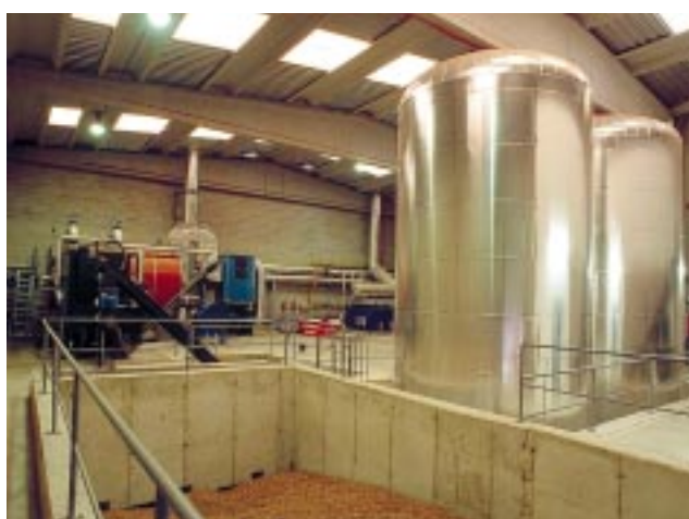
Close-up view of storage tanks, the silo and the biomass boiler in Molins de Rei plant.
