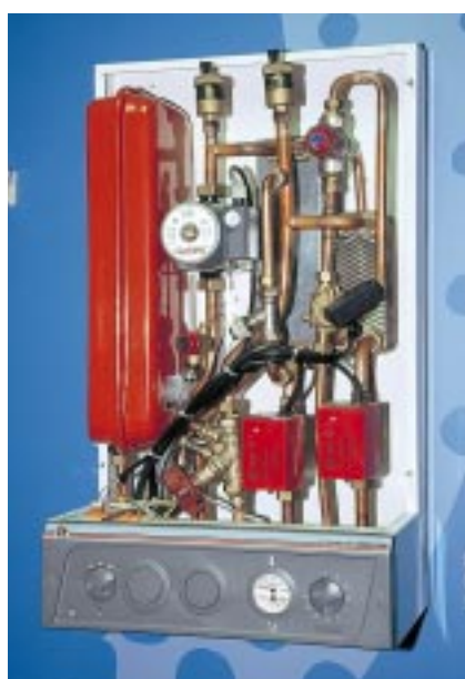
Compact facility including heat exchangers at each dwelling.
